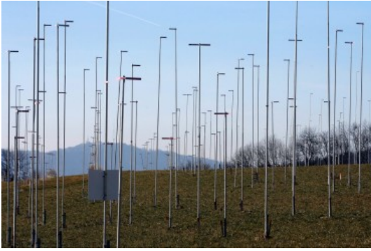
BAUGESPANN TO OUTLINE THE BUILDING VOLUME PRIOR TO THE START OF CONSTRUCTION PHOTO: ALESSANDRO DELLA BELLA, ZUMIKON, 2008
